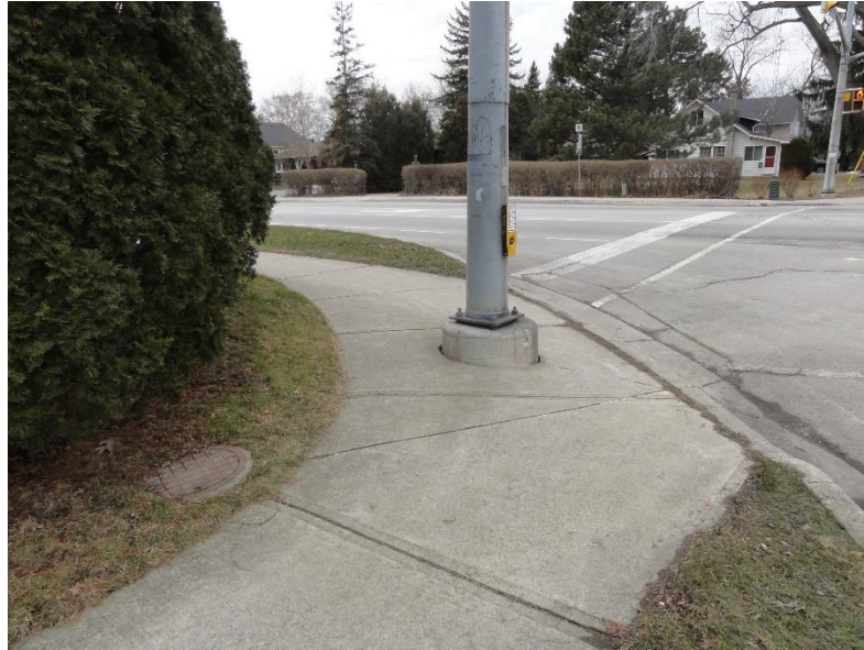
FIGURE 11: Sidewalk Too Narrow for a Wheelchair at Mississaga Street
